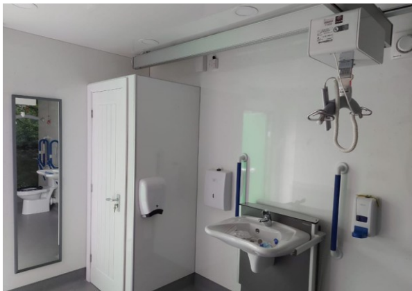
High-Spec: Both pods are finished with premium materials and specialist equipment, as per our installation at Shorne Woods park.
