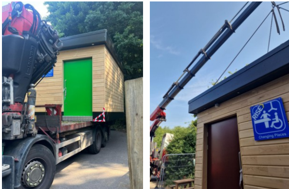
Special Delivery: Both CP Pods were delivered by hiab to Brockhill and Lullingstone as completely finished products.
