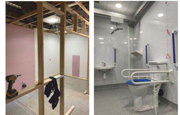
^ Before & After: We provided all building and enabling works as part of our turnkey service.
